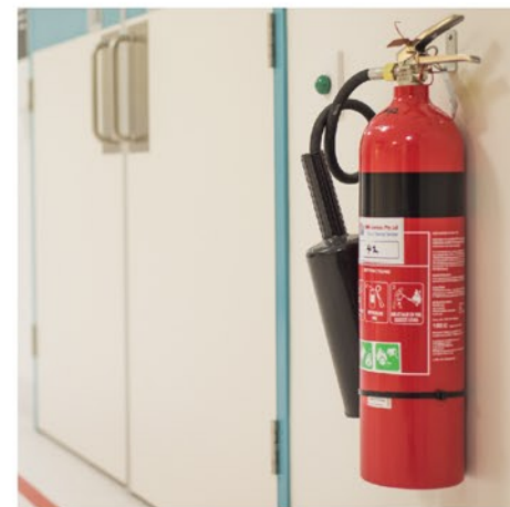
FIRE FIGHTING SYSTEMS
